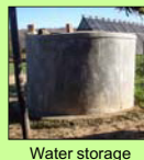
Water storage tank
